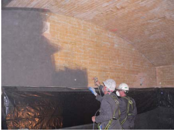
Figure 4 – Spraying EMISSHIELD® on the silica crown and silica and zircon breastwalls of an gas/oxygen-fired textile fiber furnace.
