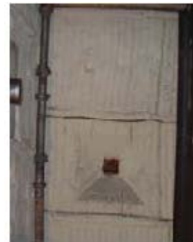
Figure 3 – Uncoated Z-Blok® after 3 months in service.
