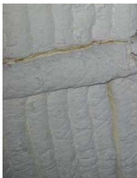
Figure 1 – Emisshield® coated Z-Blok® before start up.
