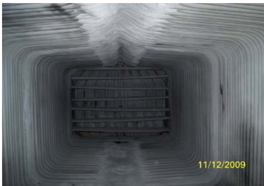
Target Wall and Tubes with Emisshield®
